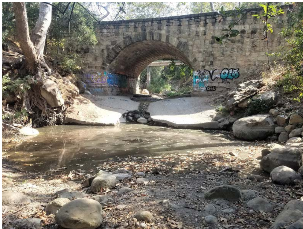
Photo 25. Plunge pool habitat and eroded apron on D/S end of Mission Canyon Road Bridge, Compensatory Mitigation Option 2 on Mission Creek. Photo facing U/S.
