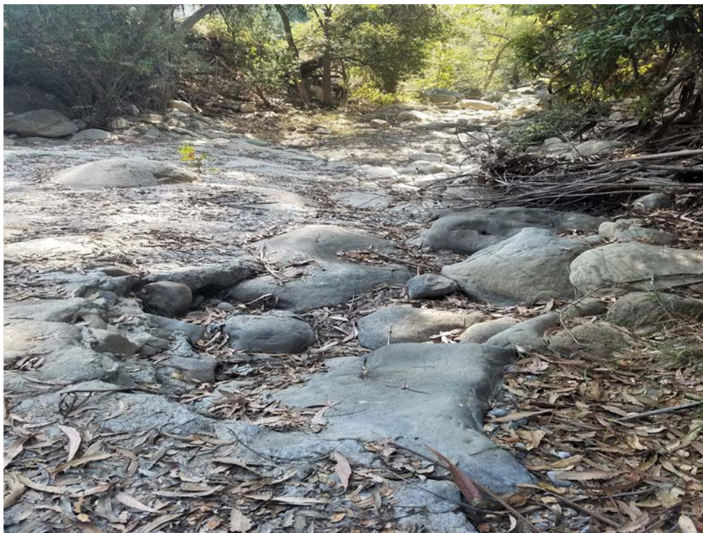
Photo 21. Wear on R side of concrete apron of the Highway 192 Bridge, Compensatory Mitigation Option 1. Photo facing D/S.
