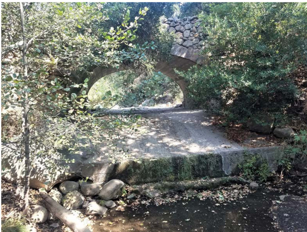
Photo 28. Plunge pool habitat and sloping apron of Las Canoas Road Bridge, Compensatory Mitigation Option 3, on Rattlesnake Creek. Photo facing U/S.
