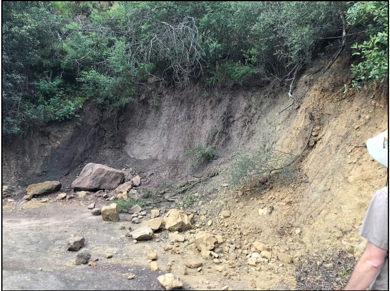
Photograph B-29. Fallen shrubs, rock debris, and topsoil; vulnerable to further erosion due to an unstable cut rock wall; photograph taken April 2020.
