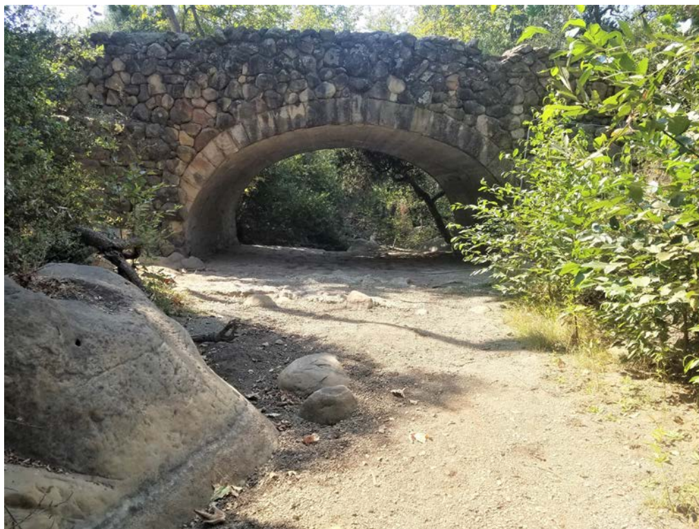
Photo 26. Las Canoas Road Bridge, Compensatory Mitigation Option 3, on Rattlesnake Creek. Photo facing D/S.
