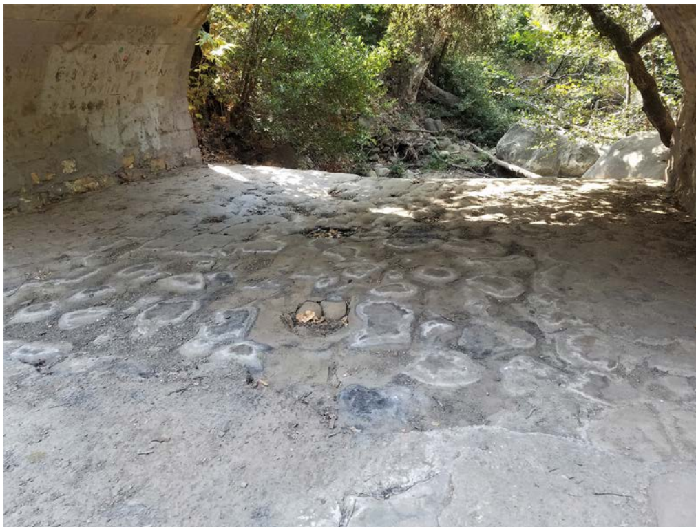
Photo 27. Flat concrete apron underneath Las Canoas Road Bridge, Compensatory Mitigation Option 3, on Rattlesnake Creek. Photo facing D/S.
