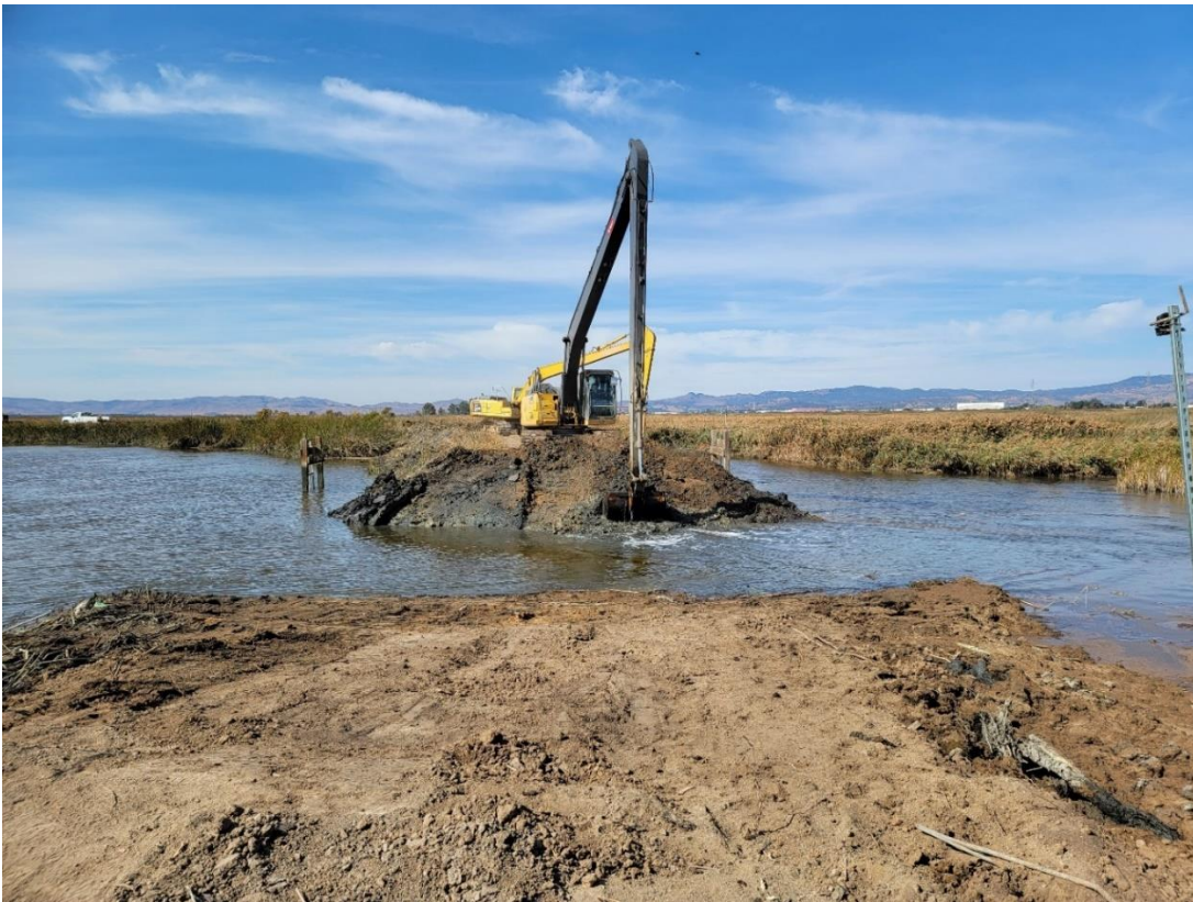
Photo 3. First breach at W5, near Grizzly Island Road Bridge.
