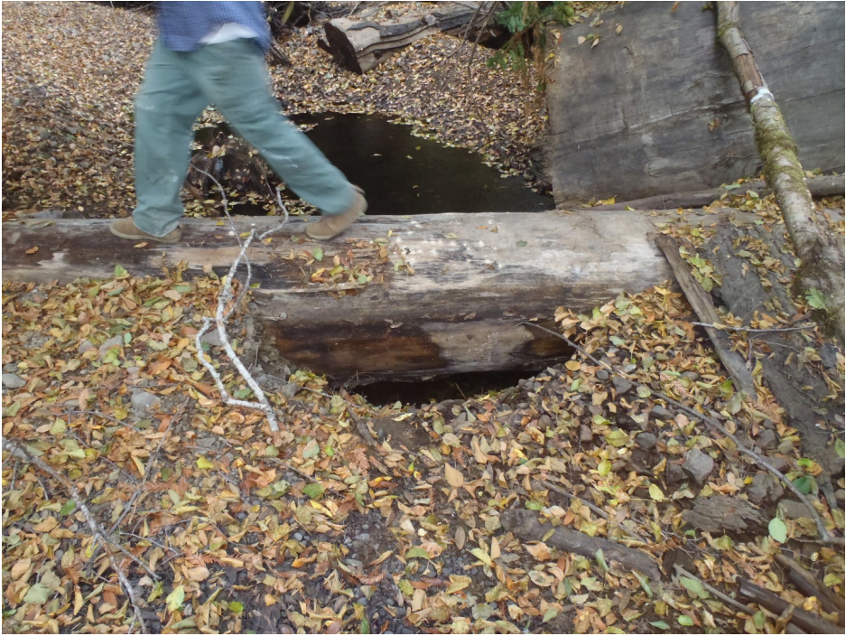
Figure 27. Log weir where the seal is broken and the flow is going under the log. Photo credit: Trevor Tollefson.
