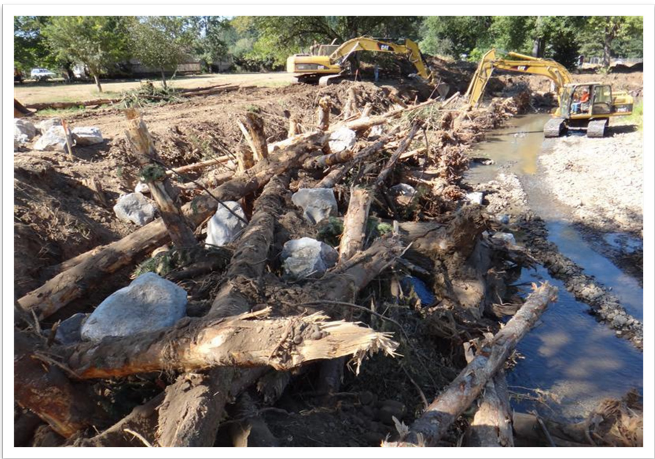
Figure 24. Combination of native streambank material, boulders, and logs used as ballast. Photo credit: Clackamas Soil and Water Conservation District.
