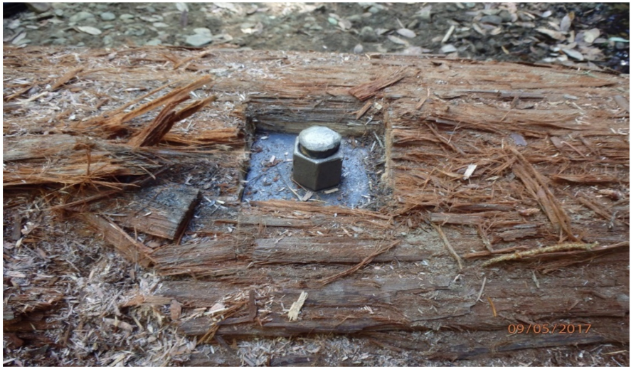
Figure 22. Finished end of threaded rebar used to secure logs together. Photo credit: Scott Monday, CDFW.
