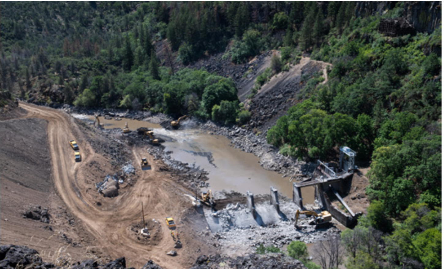
The active demolition of Copco 2 Dam in the summer of 2023, Swiftwater Films Photo.
