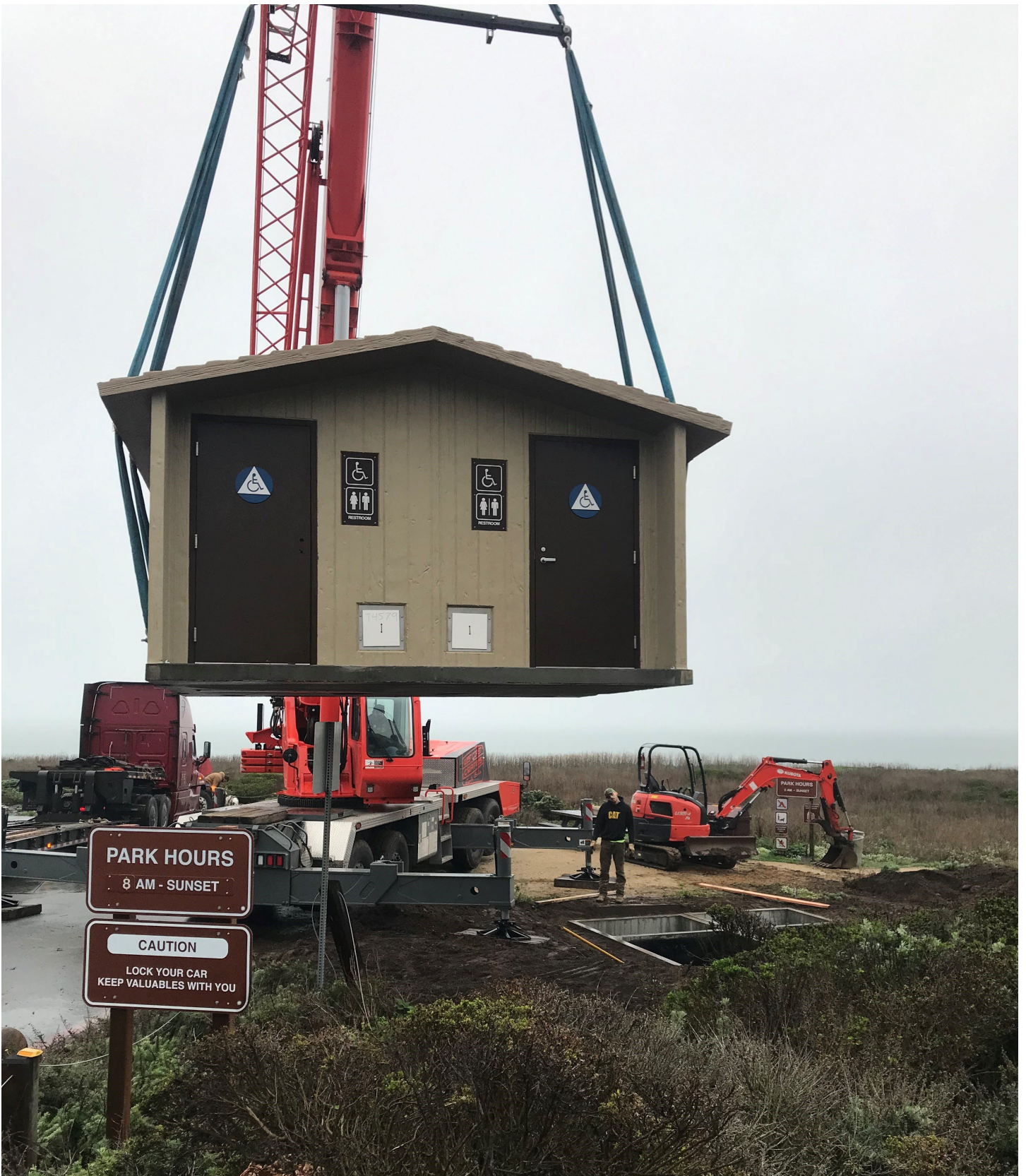
Image 3: Crane placing prefabricated restroom building on installed below ground vault. (Photo credit: California State Parks)
