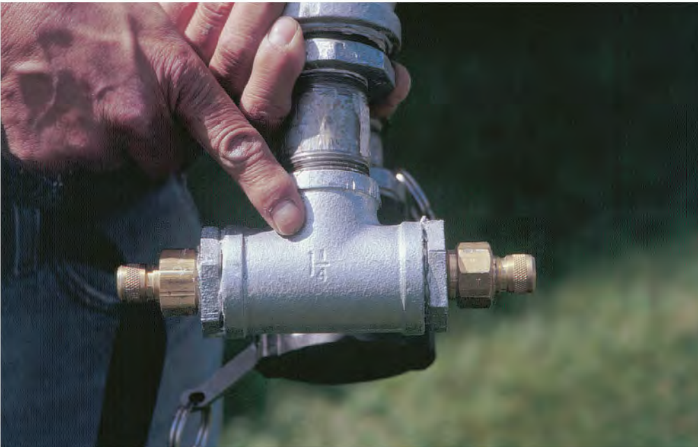
Figure C14—Garden hose quick coupler manifold.
