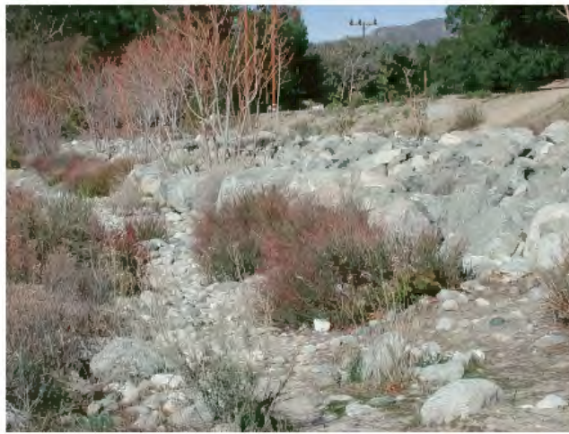
Figure 18—This area was filled to build a parking lot (flat area in upper right) and the bank was stabilized using riprap.
