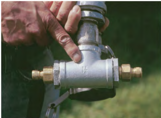
Figure C5— Garden hose quick coupler manifold.
