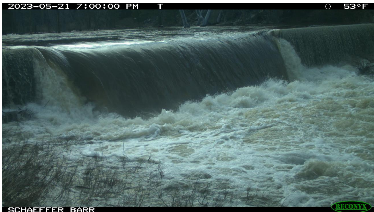
Figure 48. Picture of Schaeffer Fish Barrier documenting barrier effectiveness under peak flow conditions on May 21, 2023.
