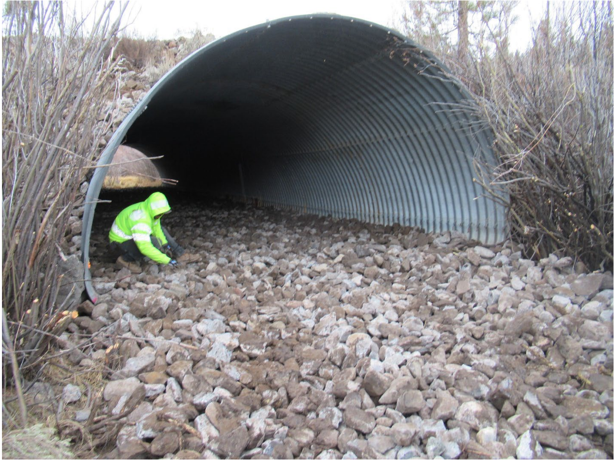
November 22, 2024 – cobble embedment placed in existing culvert to raise the base elevation.
