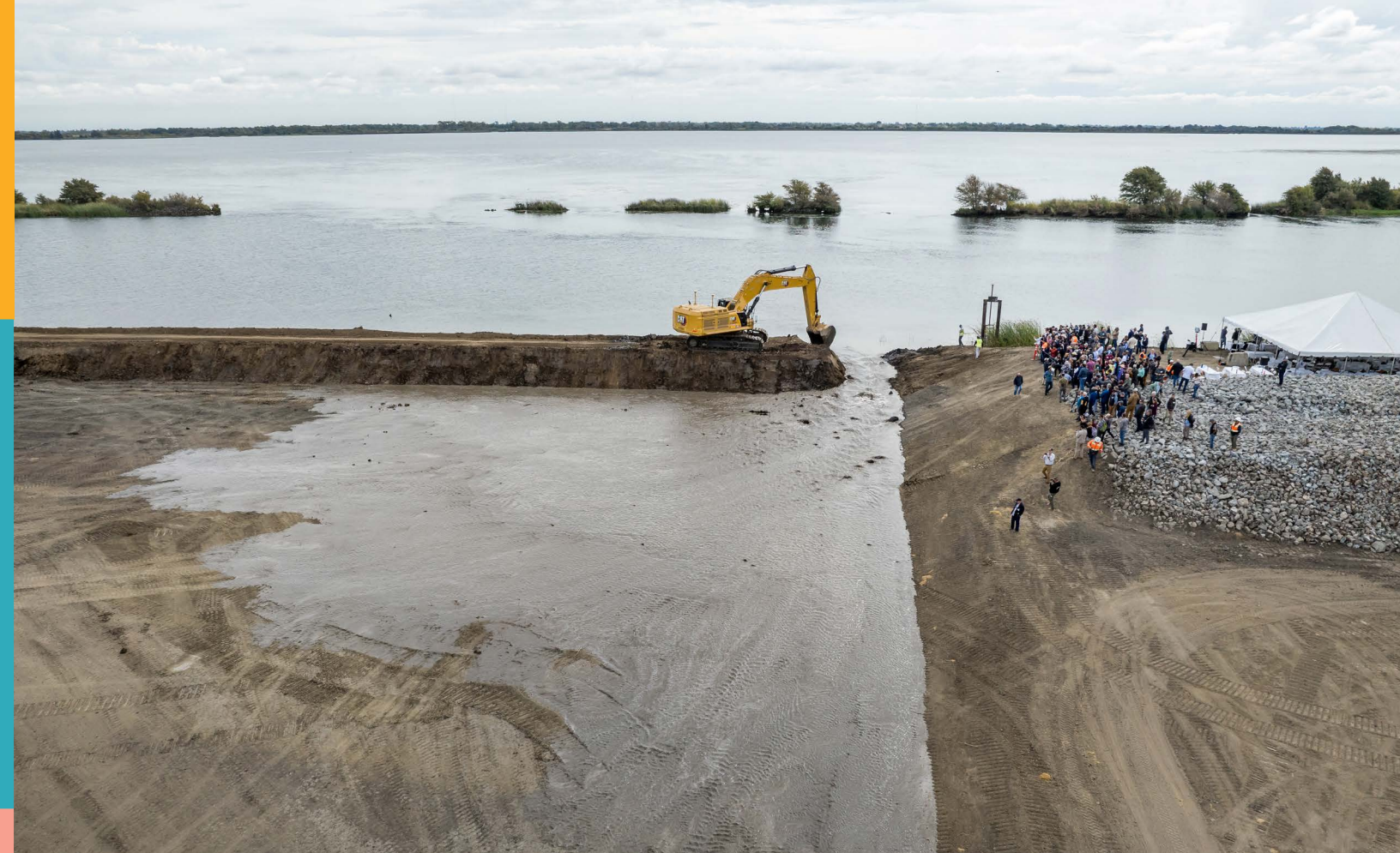
Final notching of the levee at Lookout Slough in Solano County, Credit: DWR
