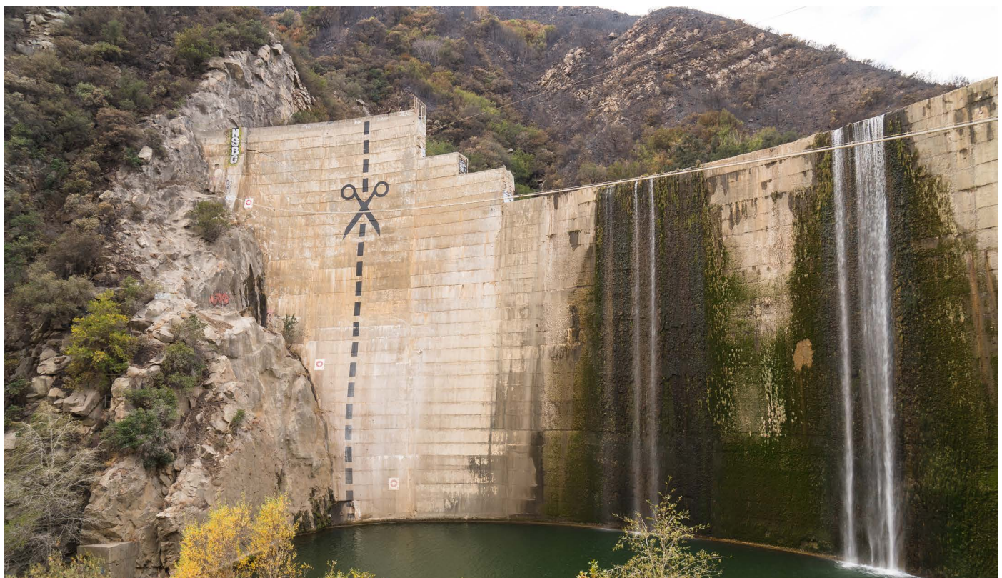
Matilija Dam on Matilija Creek, a tributary of the Ventura River, Ventura County
