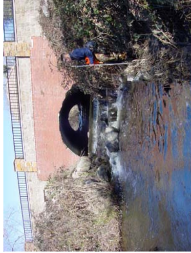
Photo 13- Culvert at Placer Canyon Road is approximately 80 feet in length, filled with rocks. May be a barrier at low flows.
