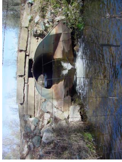
Photo 18- Culvert is perched, approximately 2 feet, and has a rusted metal apron with large holes in it. Pool below is 1 foot deep.
