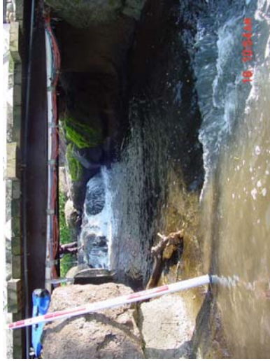
Photo 10-25 foot long concrete apron under bridge. Flashboard dam above apron requires 3 foot jump, pool has 6 inches of water in it.
