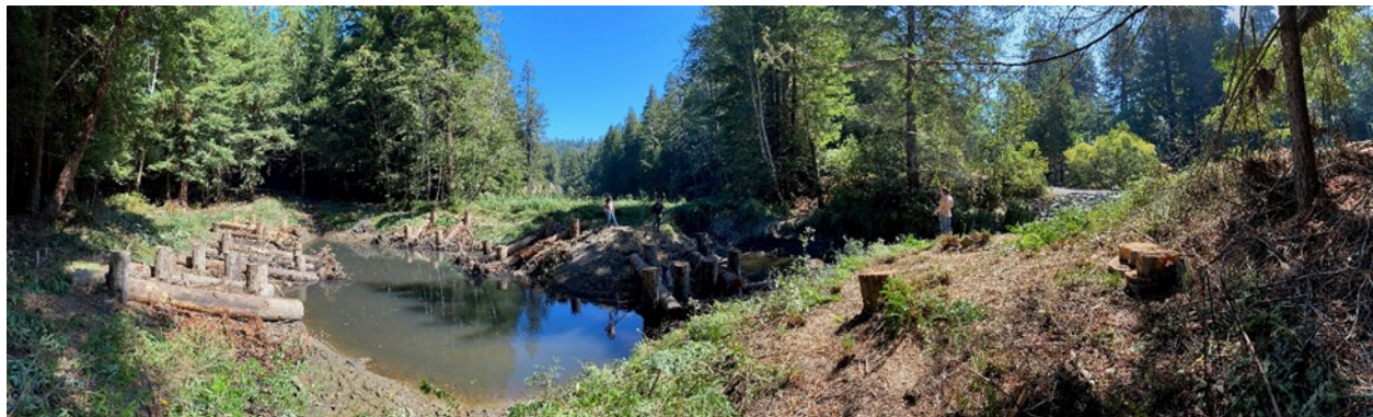
Figure 23. Culvert remediation and off-channel restoration project at Dry Dock Gulch in the Big River Estuary. Project completed by Trout Unlimited in 2023 (photo credit: Sarah Gallagher, California Department of Fish and Wildlife).
