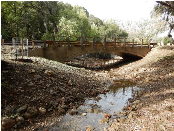
Figure 3. View, facing downstream, of the new bottomless arch culvert and upstream channel as they appeared immediately following implementation. Photo date: 1/8/2019
