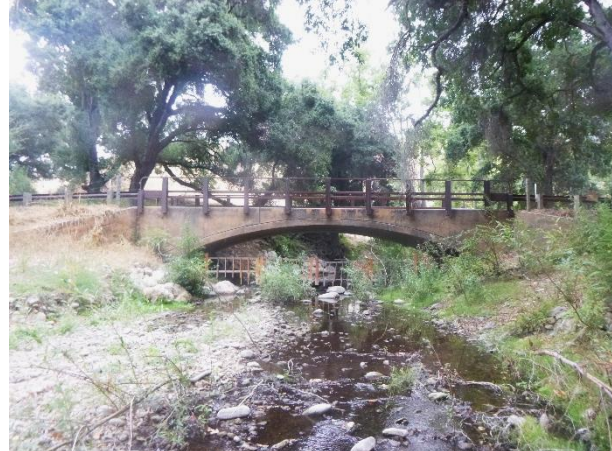
Figure 2. View, facing upstream, of the reconstructed channel and the upgraded bottomless arch culvert. Post-treatment photo date: 9/25/2023
