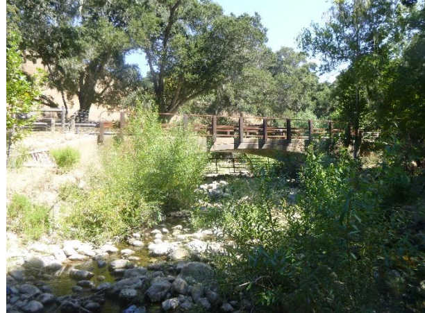
Figure 2. View, facing upstream, of the reconstructed channel and the upgraded bottomless arch culvert. Post-treatment photo date: 9/25/2023
