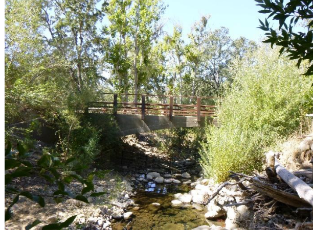
Figure 2. View, facing downstream, of the reconstructed channel and the upgraded bottomless arch culvert. Post-treatment photo date: 9/26/2023
