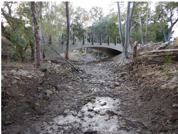
Figure 3. View, facing upstream, of the reconstructed portion of channel below the crossing with buried boulder weirs as it appeared immediately following implementation. Photo date: 10/23/2018
