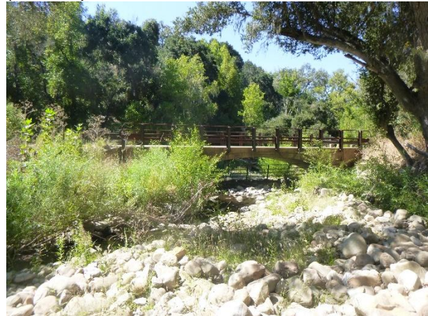
Figure 4. View, facing downstream, of the bottomless arch culvert and upstream channel, showing the shifting of the wetted channel towards river left and aggradation of substrate upstream of and beneath the crossing. Post-treatment photo date: 9/25/2023
