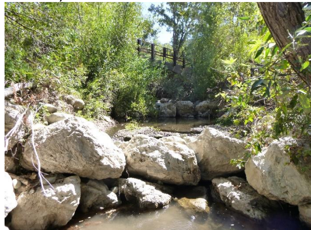
Figure 4. View, facing upstream, of the channel incision and now exposed boulder weirs in this same section of channel. Post-treatment photo date: 9/26/2023
