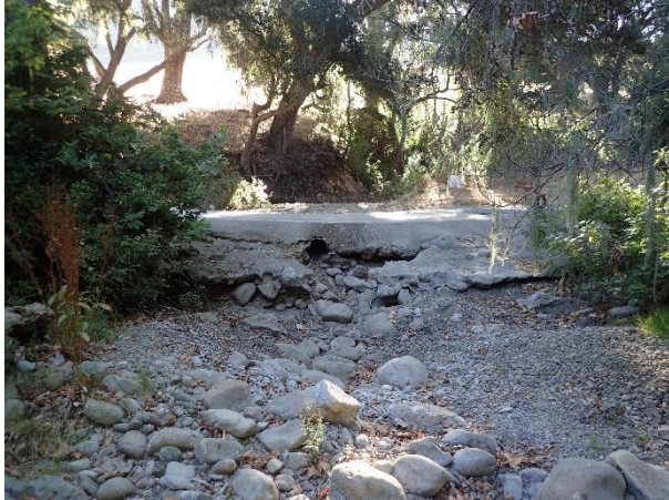
Figure 1. View, facing upstream, of the concrete low-flow crossing and the undercutting and plunge below the downstream side. Pre-treatment photo date: 7/23/2018
