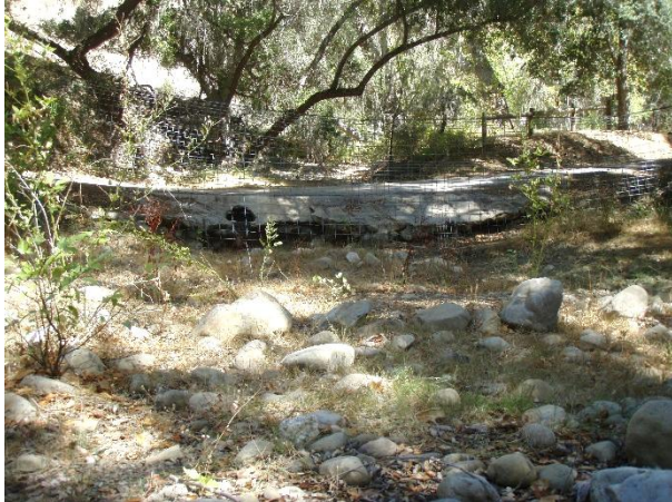
Figure 1. View, facing upstream, of the concrete low-flow crossing and the undercutting and plunge below the downstream side. Pre-treatment photo date: 9/16/2015
