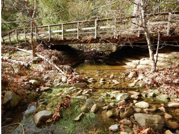
Figure 1. View, facing upstream, of the dilapidated bridge and concrete abutment lining. Pre-treatment photo date: 1/8/2019
