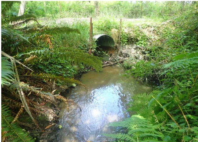
Figure 1. Upstream view of inlet to undersized culvert prior to project implementation. Pre-treatment photo date: 5/20/2021
