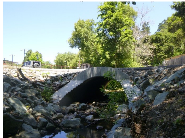
Figure 2. Facing downstream of the embedded arch culvert and reconstructed channel that replaced the previous culverts. No man-made fish passage barriers remain at this site. Post-treatment photo date: 6/5/2024
