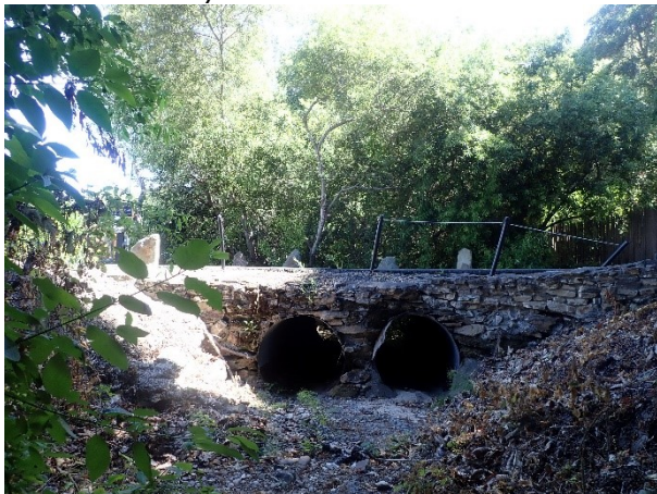
Figure 1. Facing downstream at the pre-treatment conditions of the site, showing the culverts slated for removal, which acted as total fish passage barriers. Pre-treatment photo date: 8/3/2021
