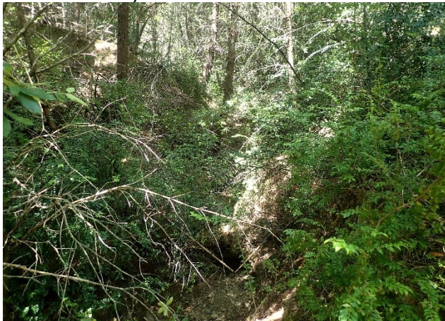
Figure 1. A stream crossing feature showing erosion and improper grade. Pre-treatment photo date: 07/14/2021.
