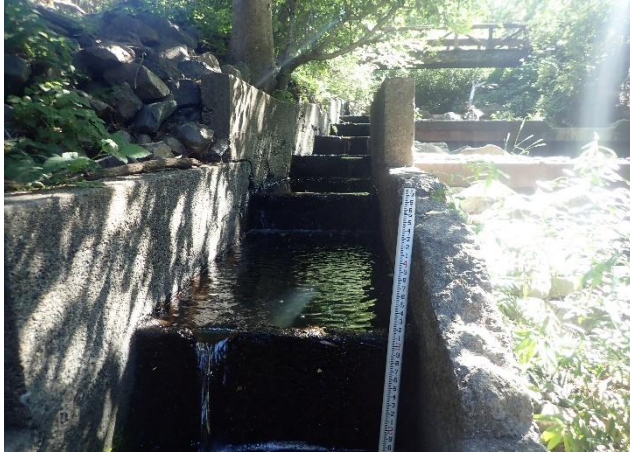
Figure 3. Concrete fish ladder next to the former dam and pools. Pre-treatment photo date: 06/30/2020
