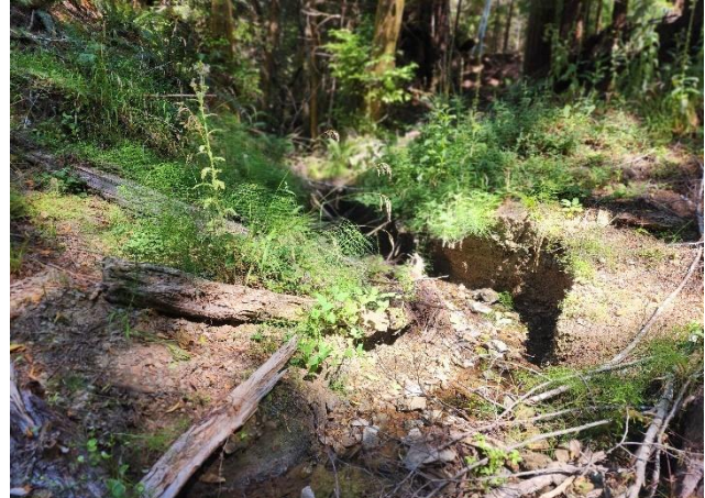
Figure 2. Excavated stream crossing, stream sides laid back at 2:1 slope. Post-treatment photo date: 07/31/2023
