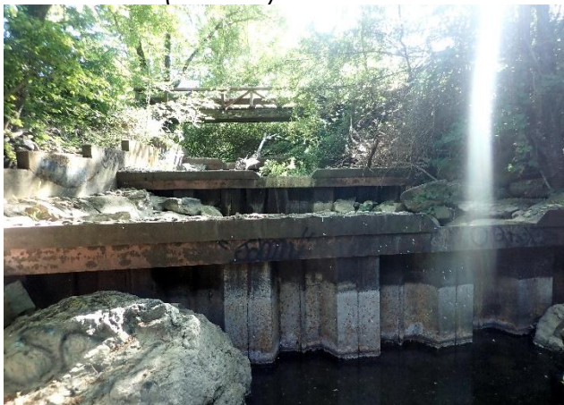
Figure 1. Concrete dams create Roy's pools with the former fish ladder on the left.
