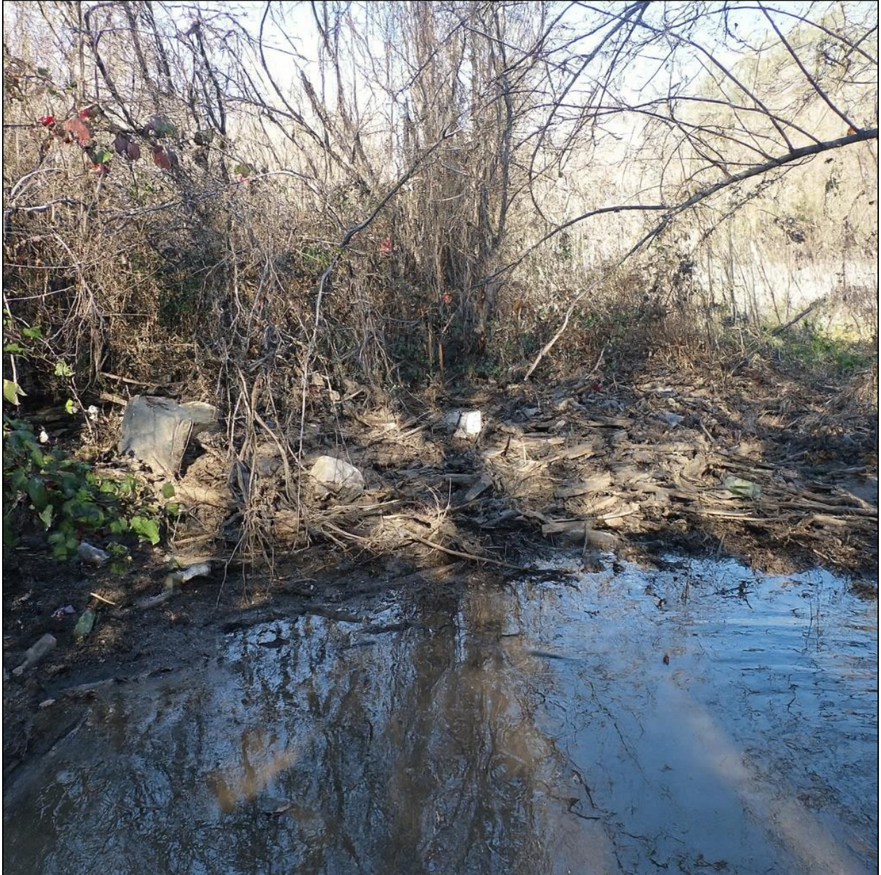
Figure 26. Artificial debris barrier located at Cole Creek near MDSA-17 at approximately 1 cfs.
