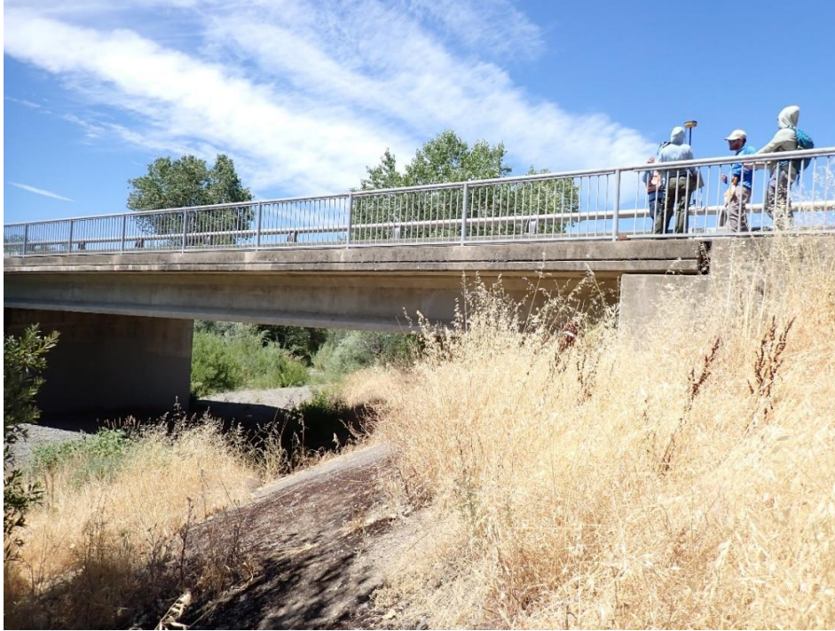
Figure 14. CDFW staff collecting instream structure measurements of Highway 20 bridge crossing on Middle Creek.
