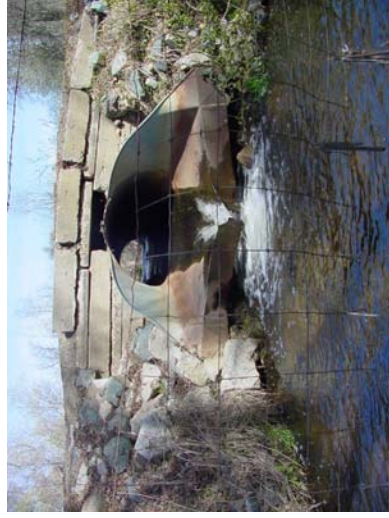
Photo 18- Culvert is perched, approximately 2 feet, and has a rusted metal apron with large holes in it. Pool below is 1 foot deep.
