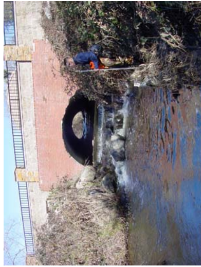
Photo 13- Culvert at Placer Canyon Road is approximately 80 feet in length, filled with rocks. May be a barrier at low flows.
