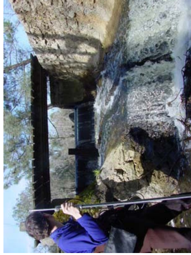
Photo17- Concrete apron is a 2.5 foot jump, pool below is 1 foot deep. Apron is 15 feet long and has 6 inches of water flowing over it.
