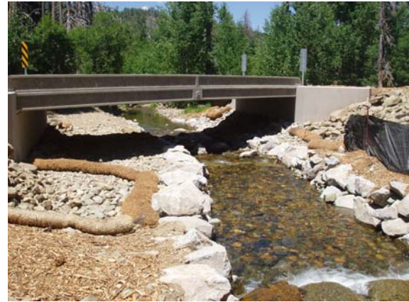
A new bridge installed as part of the restoration efforts on Tallac Creek.
