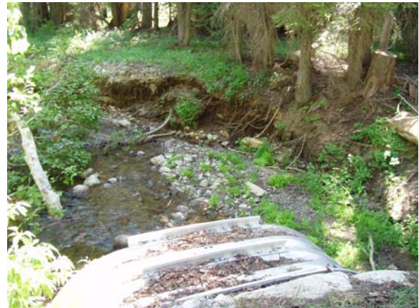
Bank erosion from an improperly aligned pipe-arch on North Fork Blackwood Creek 1
