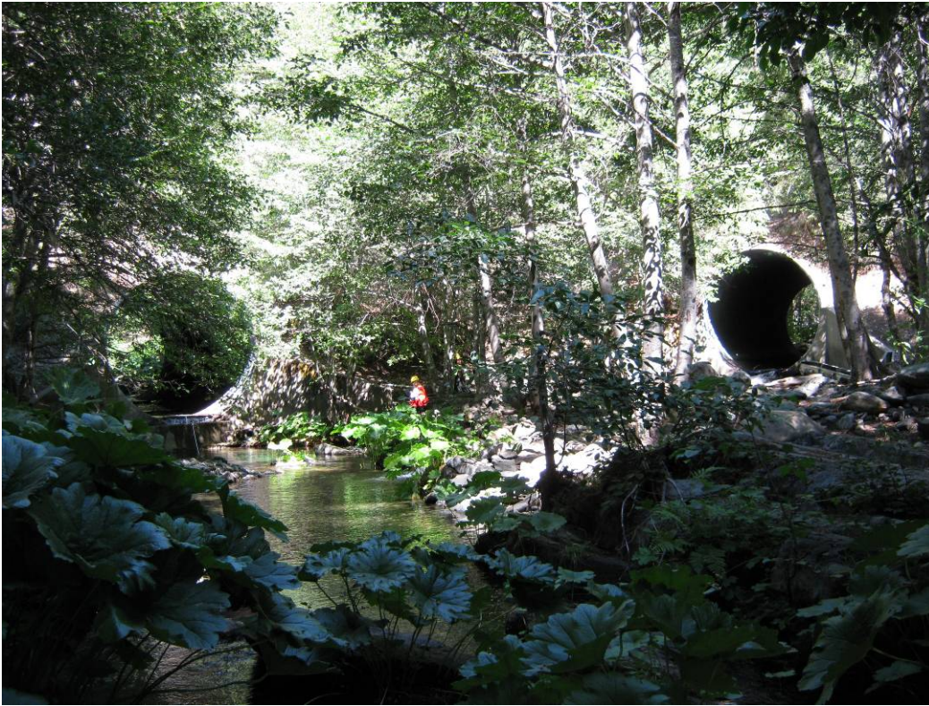
Figure 5. Twin culverts (Little Canyon Creek_1 and Mill Creek_1) crossings proposed for replacement
