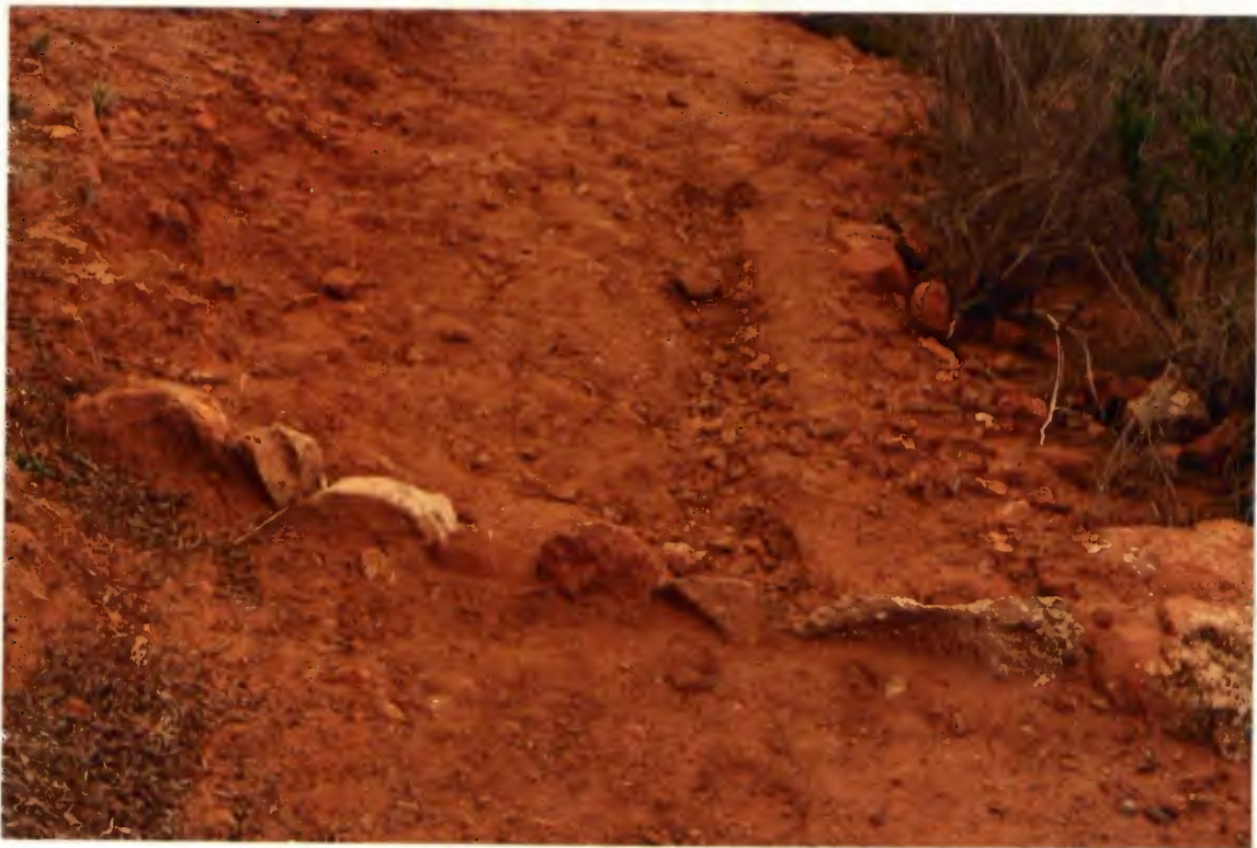
Water bars for erosion control along the trail system at McGinty Mountain Preserve
