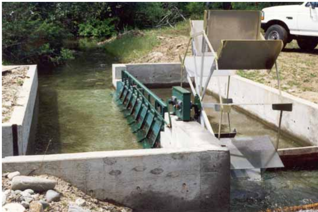
Figure 22. Lower Etna Creek diversion screen, Siskiyou County.
