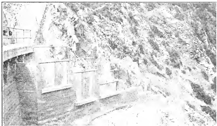
Fig. 17. Fishway at San Clemente Dam on the Carmel River in Monterey County, a fishway recently completed. Photograph by A. E. Doney.
