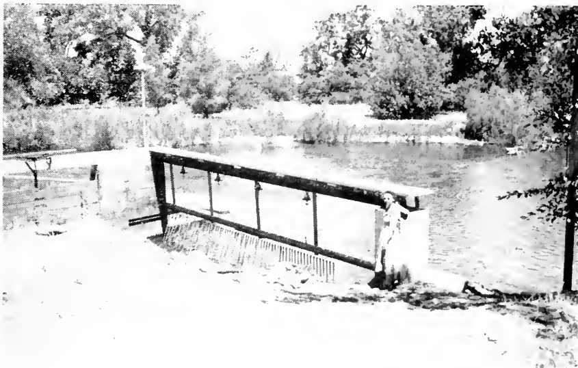
FIGURE 9. Mill Creek electric fish screen
