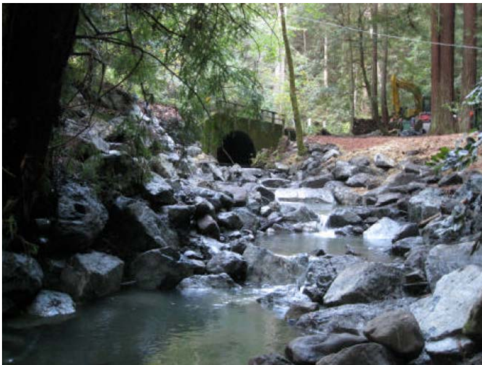
Looking upstream through the completed project area and construction of rock weirs.
