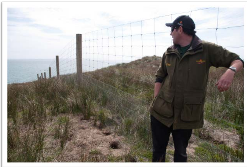
Photo 1. Martin Reid (landowner's son) looking along the new fence at a completed section. Note the rabbit digging at the edge of the mesh. The landowners patrol the fence line often checking for signs of entry and collapse any rabbit holes. The mesh 'footing' at the bottom seems
