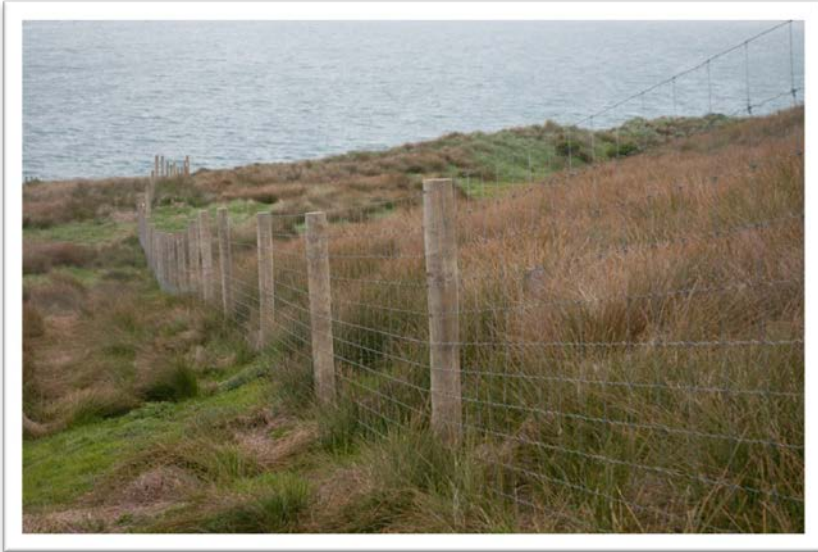
Photo 6. Partially completed section - note there is no fine mesh at the base until some way along. (photo: Jaime Newman)
