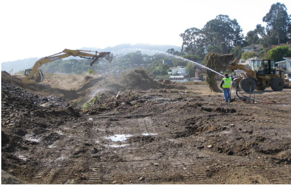
Figure 9. Contractors dig deep pits and bury large quantities of invasive vegetation including Carpobrotus edulis (Iceplant), Carduus spp. , Genista monspessulana and Phalaris aquatica
