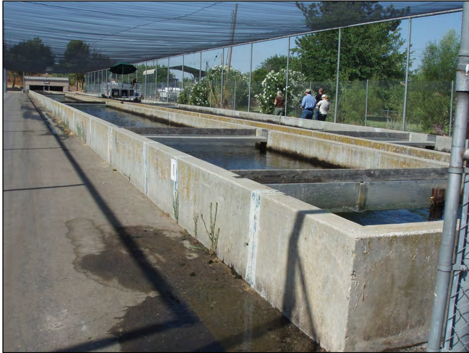
Figure 5: San Joaquin Fish Hatchery, raised concrete raceways leading to the Spawning House (Building 9), looking southwest (C. Jimenez, July 27, 2012).
