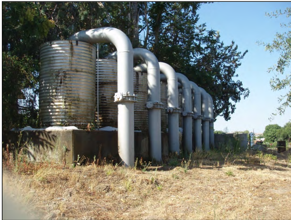
Figure 3: San Joaquin Fish Hatchery, San Joaquin River water intake, view looking south (C. Jimenez, July 27, 2012).
