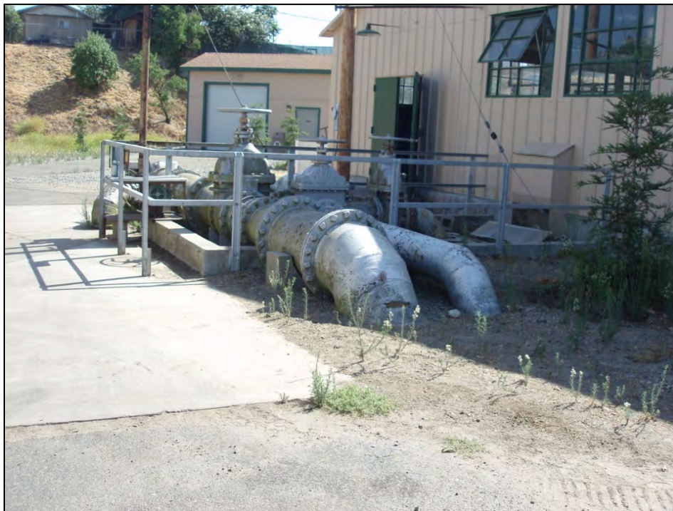
Figure 4: San Joaquin Fish Hatchery, water pipe outlet leading to other hatchery buildings, view looking north (C. Jimenez, July 27, 2012).
