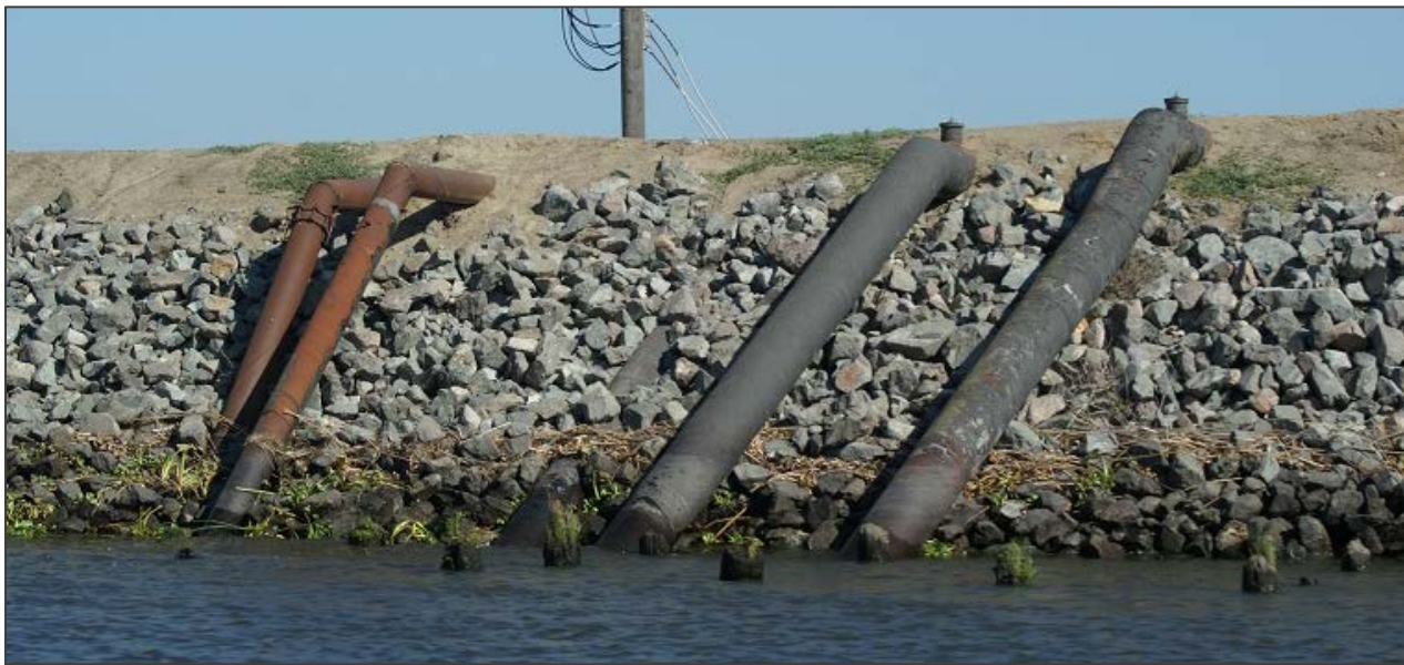
Water diversion pipes in the California Delta
