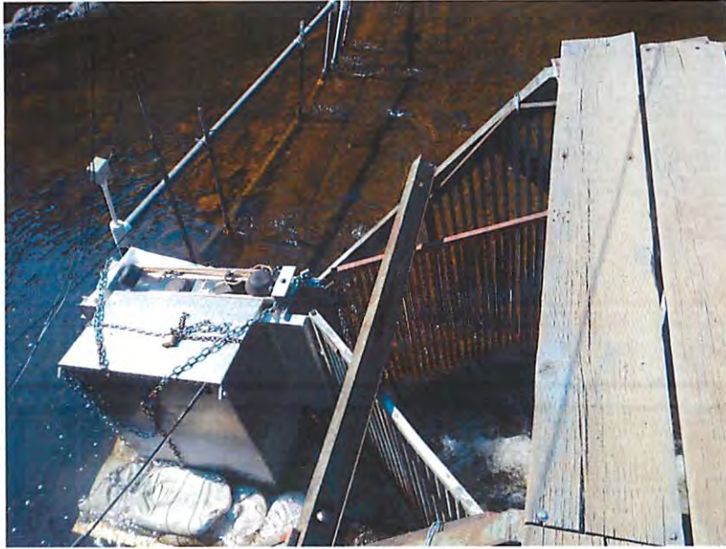
Figure 2. Camera housing and flume, SRFCF.
