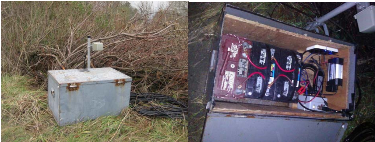
Figure 6. Left bank DIDSON power and communication box showing configuration of the batteries, inverter, topside box and wireless router (right) and antenna (left).
