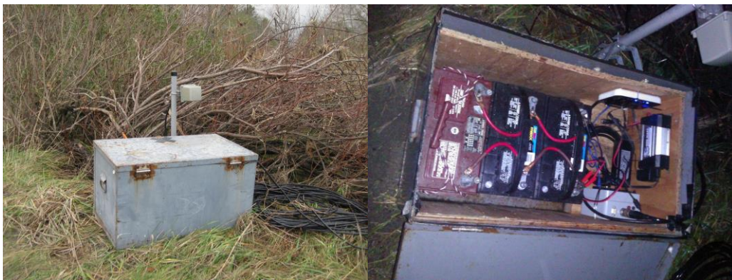
Figure 4. Left bank DIDSON power and communication box showing configuration of the batteries, inverter, topside box and wireless router (right) and antenna (left).
