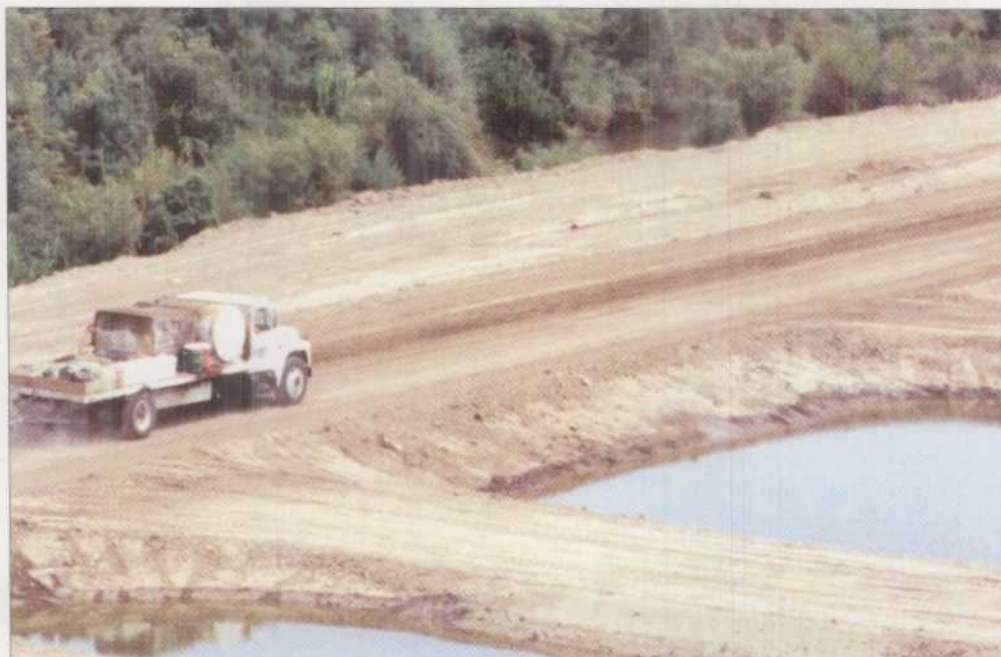
Manmade wetlands, like this one which was constructed along the New River, are one option for improving water quality.
