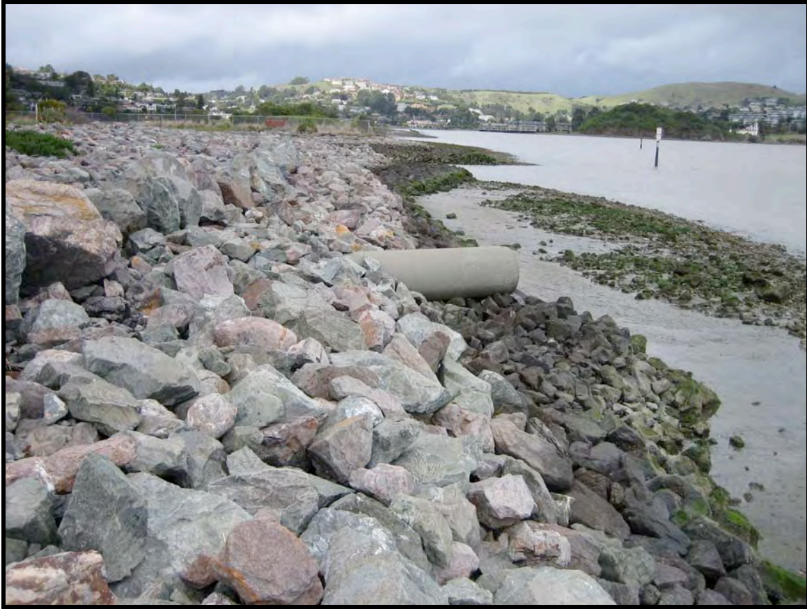
Photograph H. South end of Strawberry Point (looking north) is devoid of habitat.
