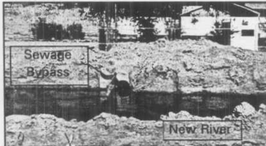
Figure 203 - Bypass from Lift Station into New River (Jan 1998)
