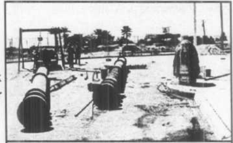
Figure 176: Work underway to correct problems at Pumping Plant No. 3 (formerly PP1A) (Aug 1995)
