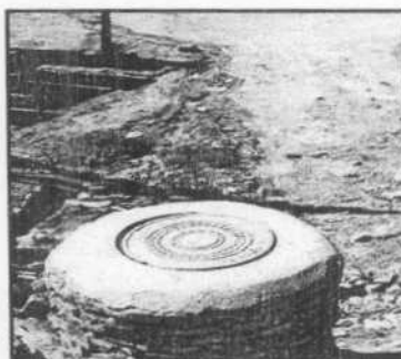
Figure 91: Overflowing sewer manhole (Apr 1988)
