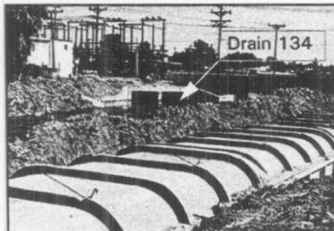
Figure 198 - Drain 134 discharging into the New River (Mar 1998)
