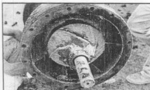
Figure 90: Replacement of worn pump at Pumping Plant No. 1 as part of joint U.S./Mexico $1.2M project (Feb 1988)
