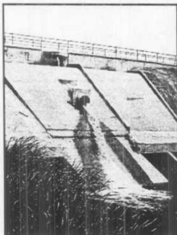
Figure 140: Bypassing of raw sewage from South Collector (Apr 1994)
