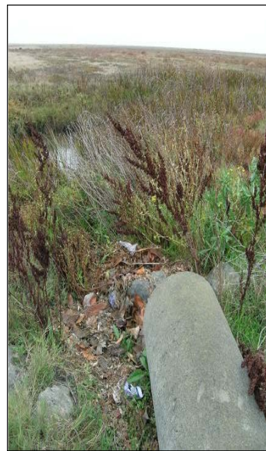
Trash at culvert outlet, White Slough Unit
