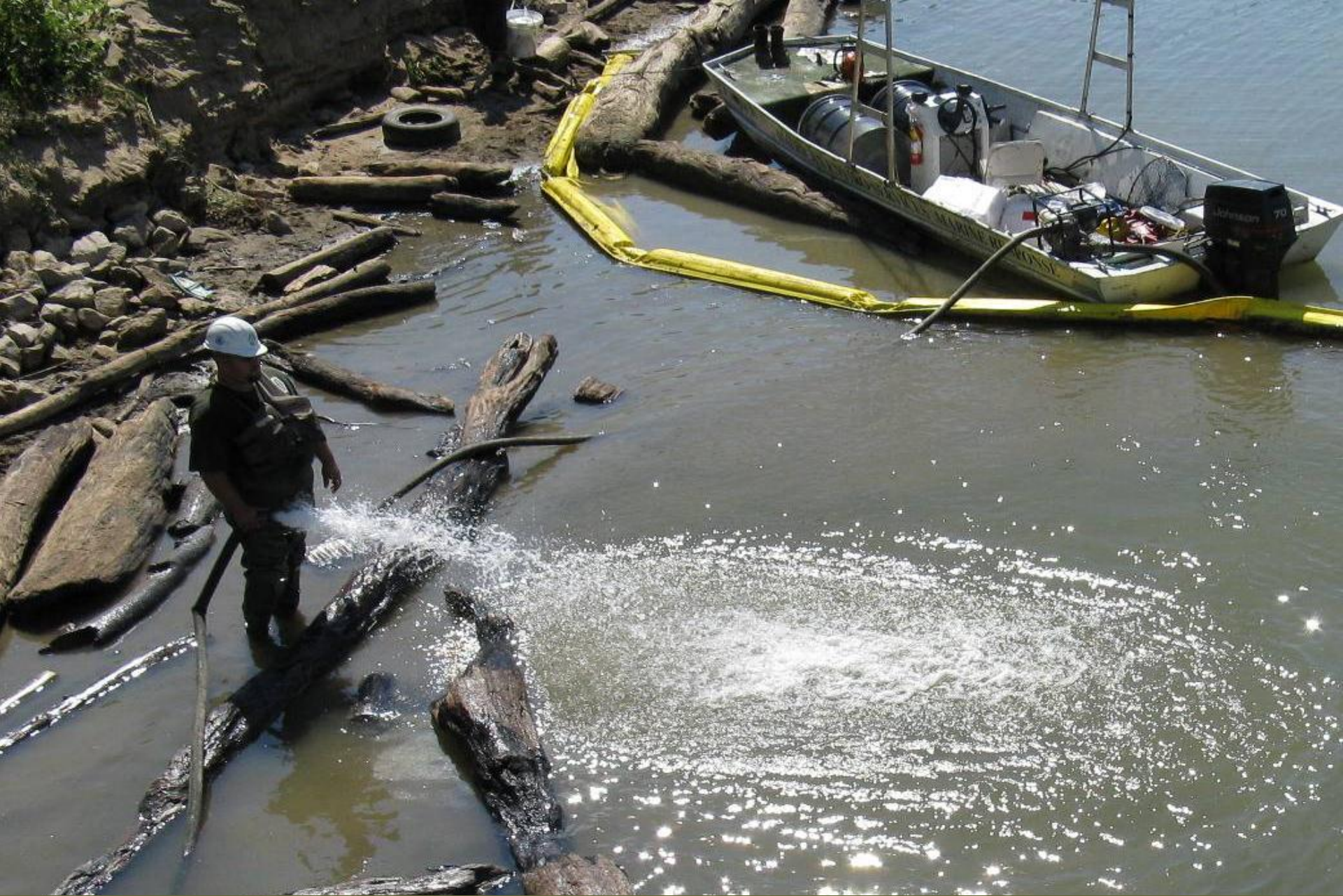
Using low pressure water to push solidified material to collection area.
