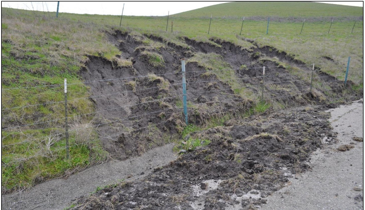
Photo 10: View of natural erosion issues uphill of access road. Hillside sediment sloughing into road.
