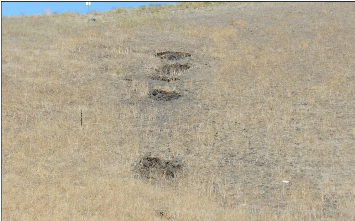
Photo 4: Closer view of sink holes, looking northwest
