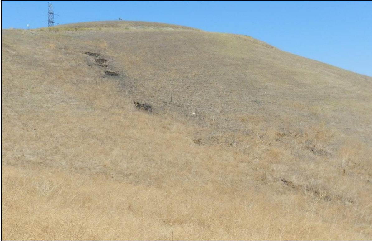
Photo 3: View of sink holes, looking north (North Dublin Transition station in far left background)
