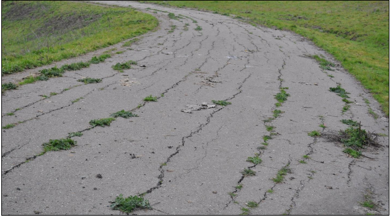
Photo 9: View of road surface cracks along lower 1/3 of road alignment.
