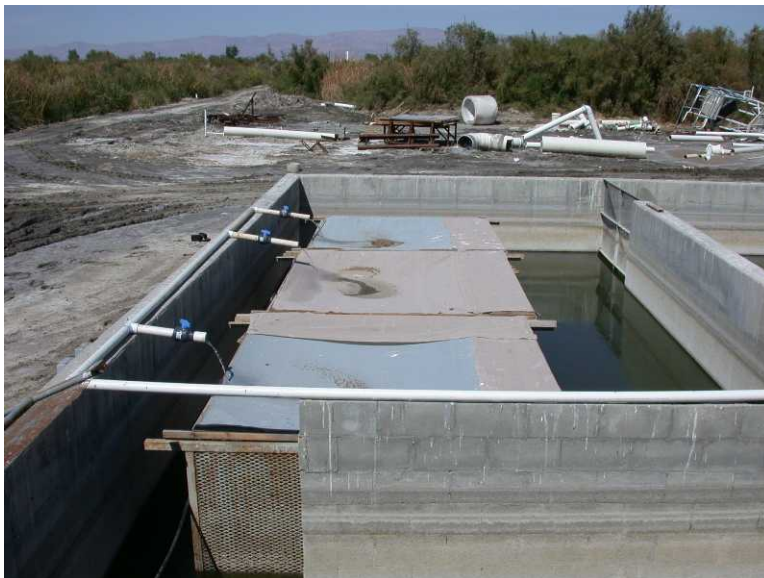
Photo 4. The drained CEP algal harvest section with sedimentation belt. Photo 4.
